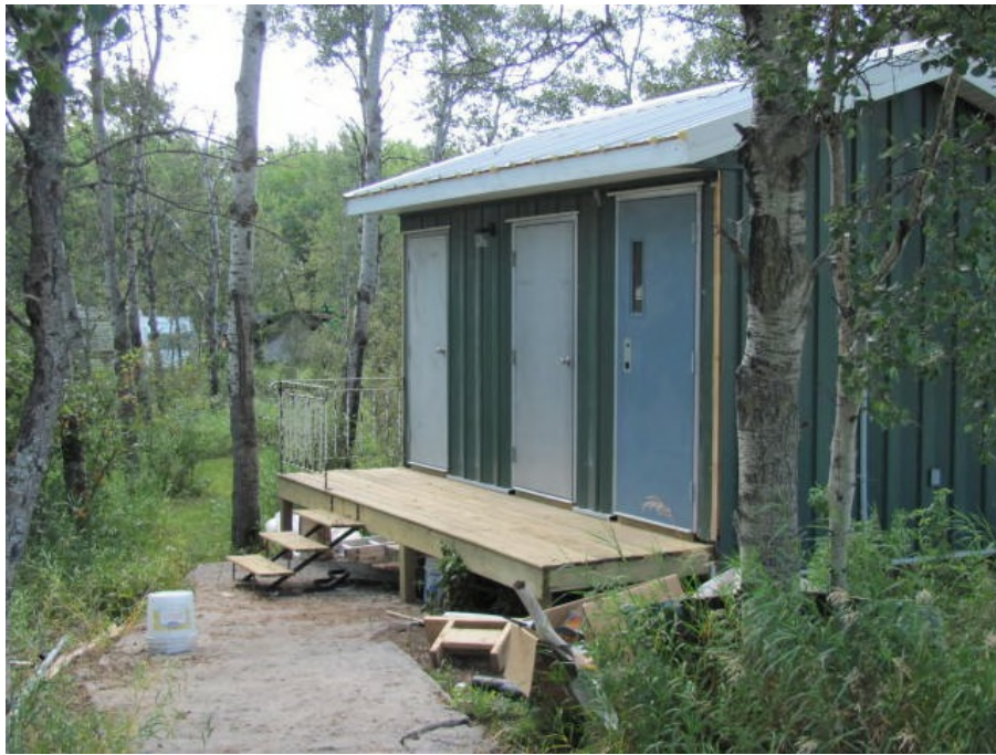
New CLUB Outhouse Running Water and Flush Toilets
